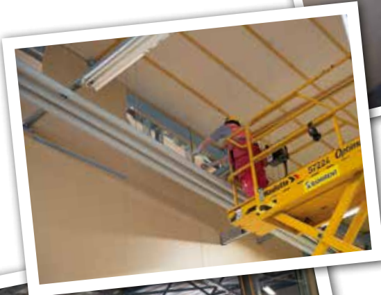
...sometimes they measured and fitted plates in place just below the roof.
