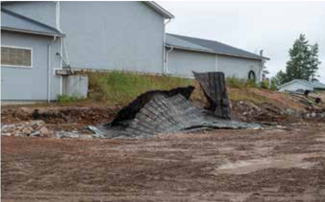
The protective safety cover just jumped when a last 10kg blast finished the excavation for the foundation of Darekon's new building.
